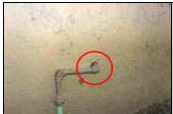
Look for gaps around pipes outside your home
