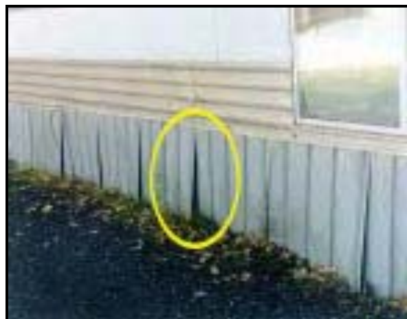
Fix gaps in trailer skirtings
